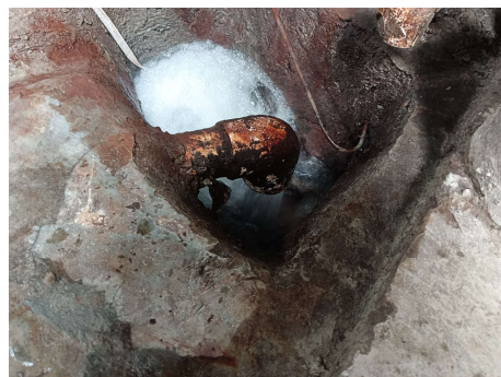
Discharged wastewater [15/11/2024, 12:30 PM]
